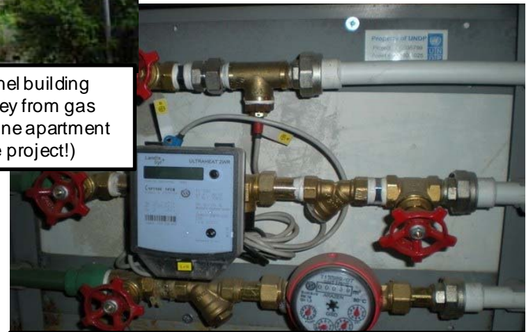
Heat meter installed at the entrance to an apartment in Avan district of Yerevan
