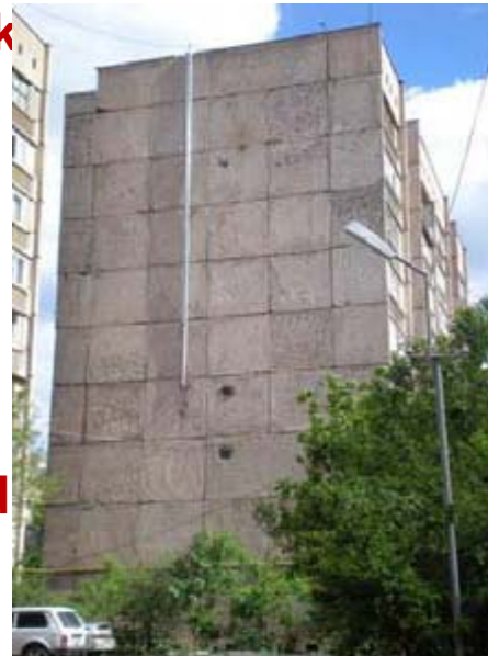
Multi-apartment panel building with exhaust chimney from gas heater installed in one apartment (not financed by the project!)
